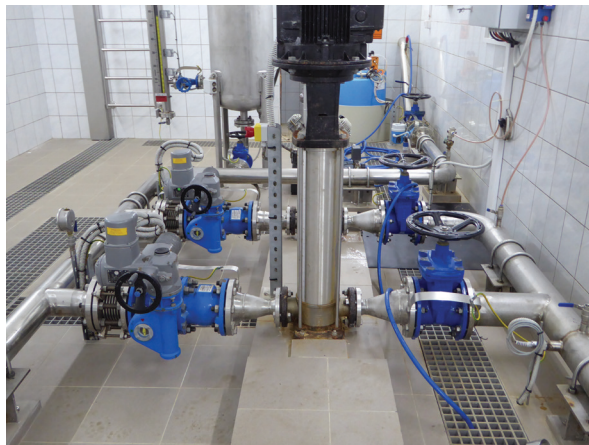
Photo 5: The pumping room
